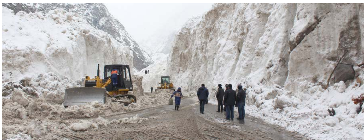
Rehabilitation of traffic movement on the Dushanbe-Khuand highway after the descent of the avalanche
